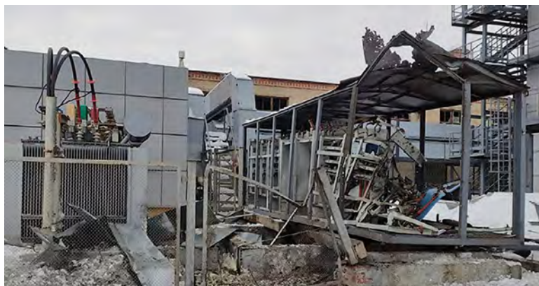
▲ A neutron source substation at Kharkiv Institute of Physics and Technology destroyed by Russian attacks on 6 March, 2022. © State Nuclear Regulatory Inspectorate of Ukraine.
